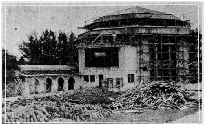
—Daily News Photo by Kolsbun Workmen Saturday began removing the last exterior forms from the Bryan Memorial church, Coconut Grove. The church, which was to have been named the Grove Temple, is located on the grounds of the late William Jennings Bryan, just west of Marymont, the Bryan estate on Biscayne bay.
