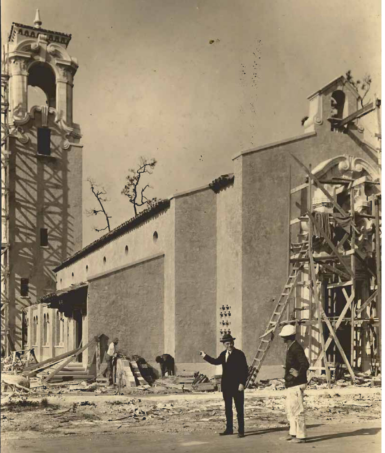
Richard Kiehnel on site during construction of Coral Gables Congregational Church (1923), 3010 DeSoto Boulevard, c.1923. (Office of Historical Preservation, City of Coral Gables)
