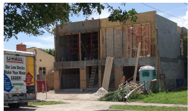
Figure 3.83: Current photograph (2019) of the duplex under construction at 1120 SW 13th Avenue (source: Plusurbia Design).
