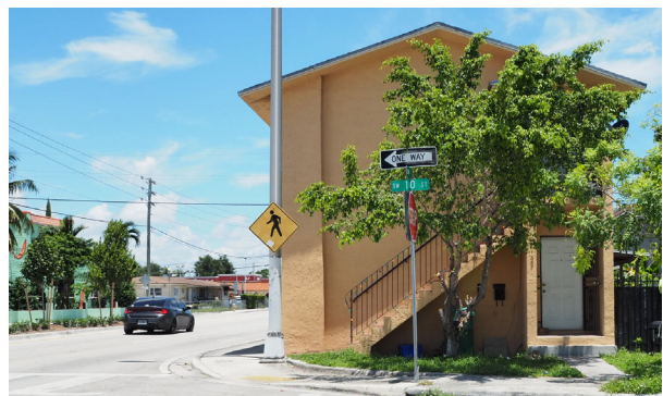
Figure 3.76: Current photograph (2019) of the building at 1687 SW 10th Street. The entire front facade, including the shaped parapet, decorative roof tiles, medallions, and front arched entryway were removed to accommodate the widening of 17th Avenue (source: Plusurbia Design).
